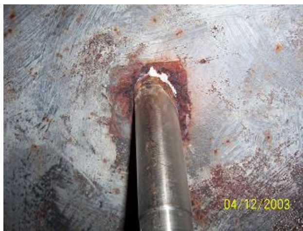
Figure 2. Reactor vessel bottom mounted instrumentation nozzle.
