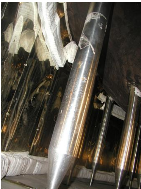
Figure 4. Duct tape residue
