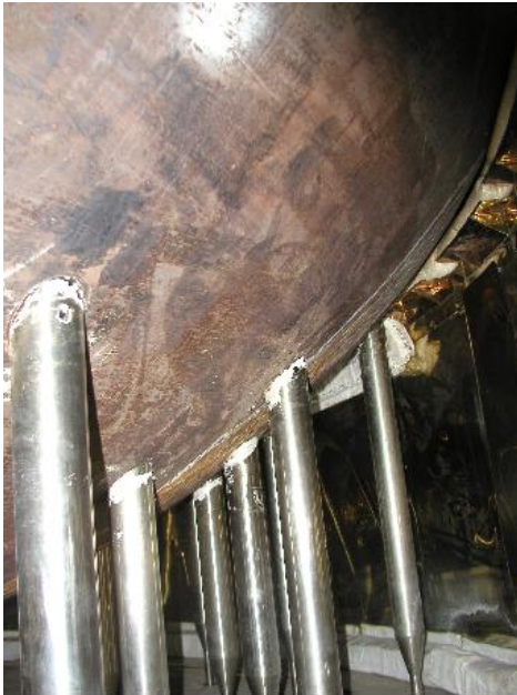
Figure 3. White paint on BMI penetrations
