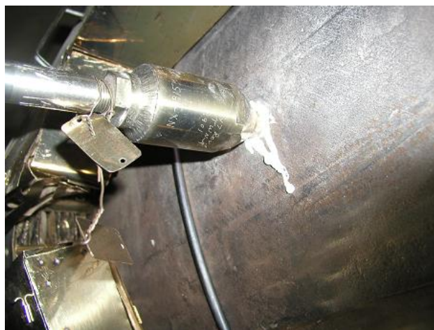
Figure 1. Hot leg instrumentation nozzle with boric acid deposit.
